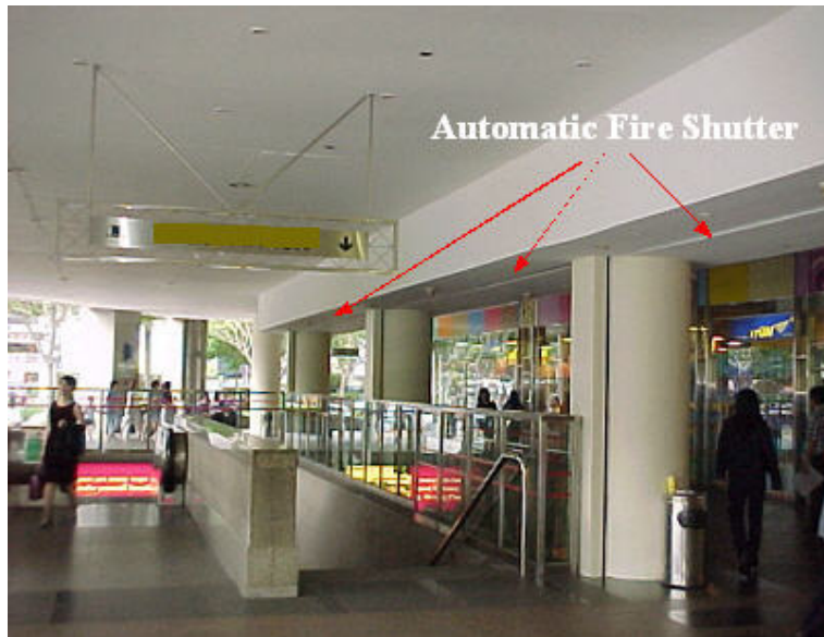
Figure 4-35 An automatic fire shutter at the interface between a commercial development and station entrance
