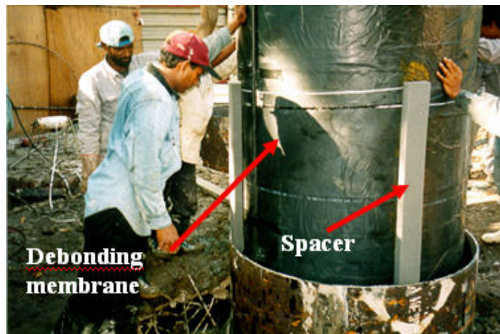
Figure 3-10 Spacer provided to prevent the debonding membranes from any damage during installation
