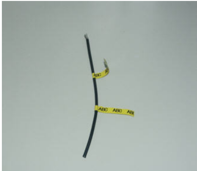
Figure 5-3 Tagging of cables for identification of monitoring company & development project
