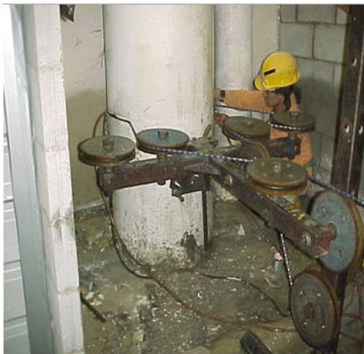
Figure 2-14 Use of a diamond wire saw for cutting station structure helps to minimise vibration and noise levels
