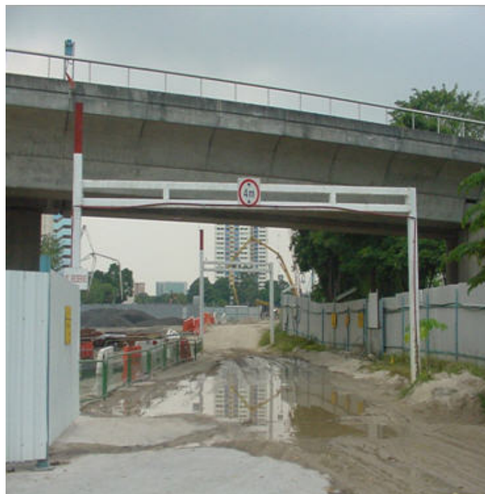
Figure 2-10 Temporary height restriction gantries are provided on both sides of the viaduct beam
