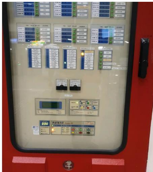
Main Alarm Panel
